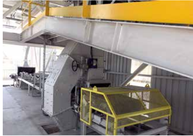
Ciner Group / Denmark Derince Ship Loading Project, Mechanical Works (Basic & Detail Design + Supply + Installation)
