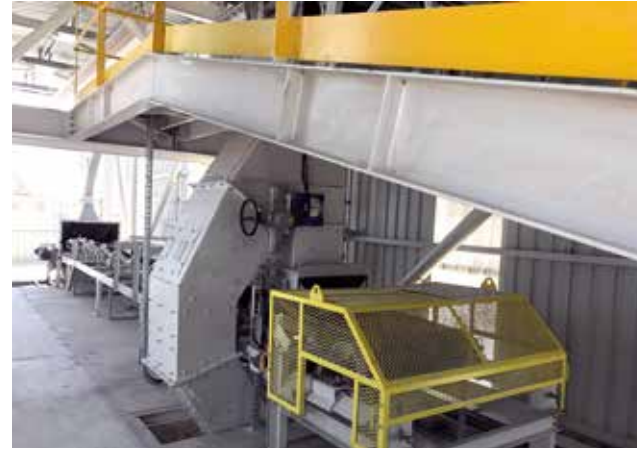
Ciner Group / Denmar Derince Ship Loading Project, Mechanical Works (Basic & Detail Design + Supply + Installation)
